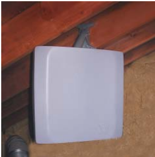
Attic mount on overhead rafter.
